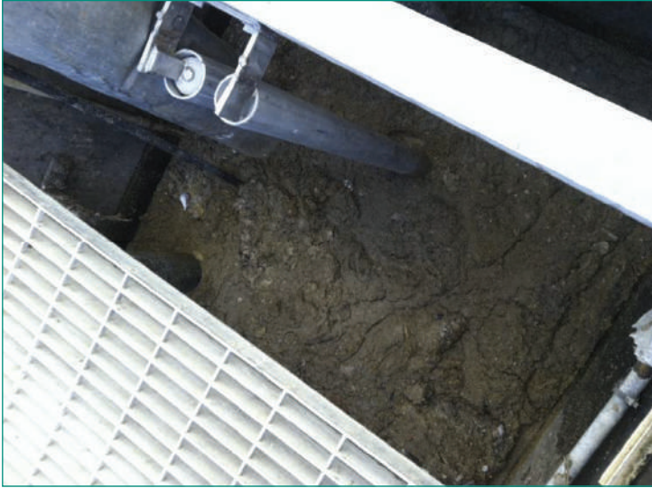
Fig. 1: With the grate open, a 2 - 3 foot grease layer is evident prior to treatment.
